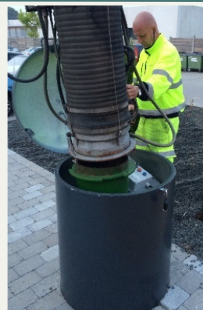
Figure 32 - Emptying raised suction stand
